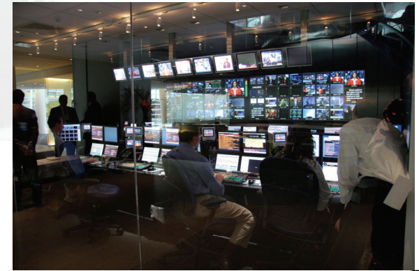
CEI DESIGNED PRODUCTION CONTROL CENTER—NEW YORK
