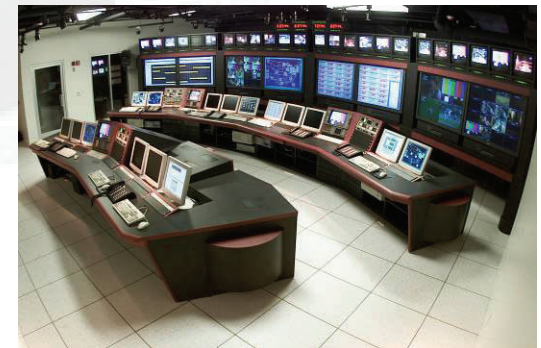
CEI DESIGNED FOX NETWORK OPERATIONS CENTER
